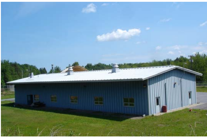
The metal roof of this DOT Building, approx. 20 years old, has been renewed with the MRR System from Roof-Tek®. The leaks have stopped, and the entire building looks like new.
