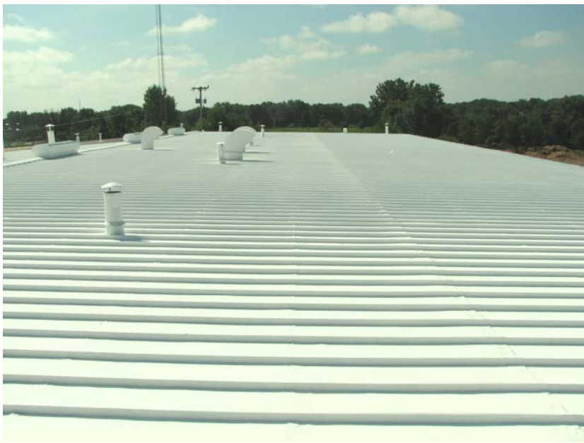
This metal, panel roof has been renewed with a sustainable, elastomeric coating system, MRR - Metal Roof Restoration.
