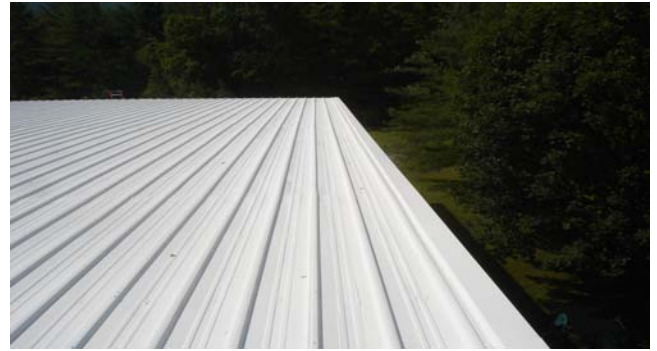
An existing metal roof can be made to look and perform like new; rust, leaking seams and fasteners will be repaired before the application of attractive, new topcoats.
