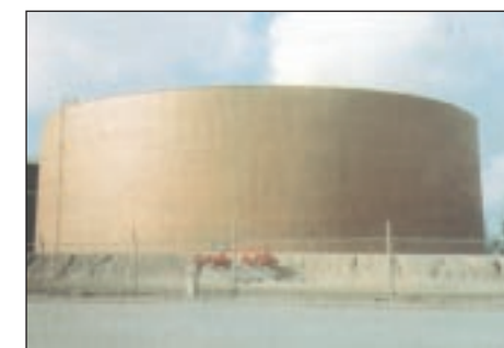
A petroleum storage tank on the Gulf Coast is insulated and protected by BaySystems spray foam.
